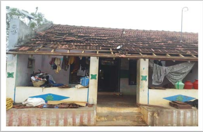
Damages to the dwelling places
